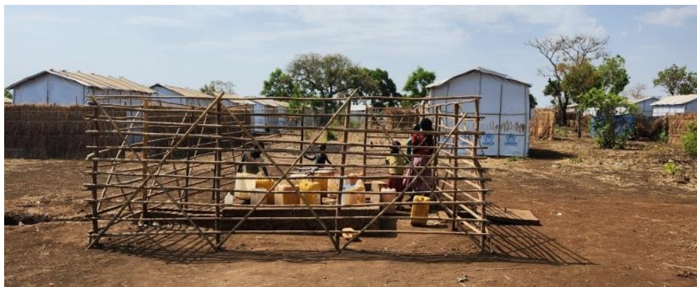
Water point in Ura Settlement.
